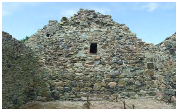
Kilbroney Medieval Church, Rostrevor: Cintec anchors installed to consolidate the leaning west wall of the medieval church ruins.
