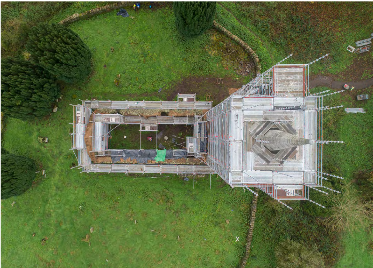
Above: Conservation work in progress at Church Island State Care site, November 2022.
