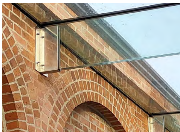
Templemore Baths, Belfast. Glass roof supported on glazed fins provides light touch intervention between historic building and new extension.
