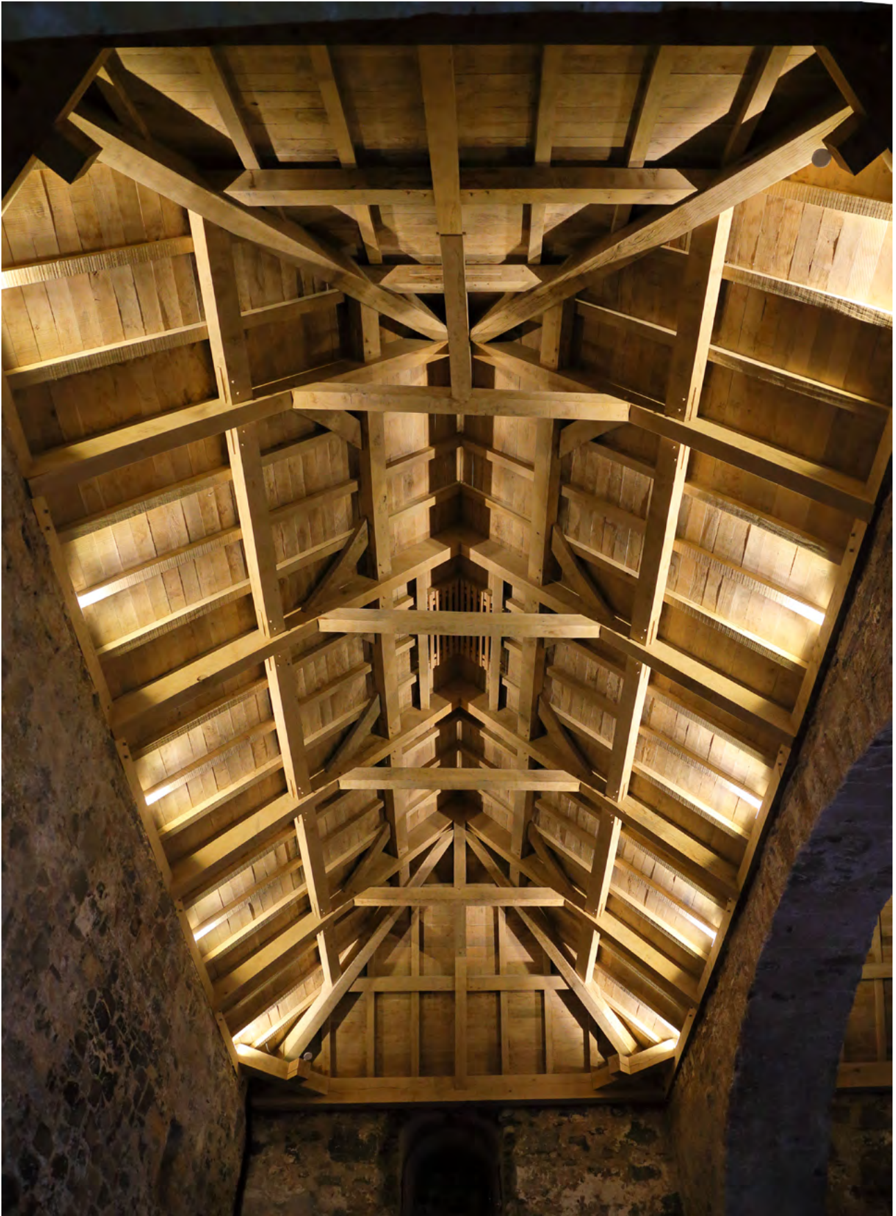
Above: Interior view of the new Irish oak hipped roof structure over the Great Hall, Carrickfergus Castle, replacing an earlier 1930's flat roof. A dedicated team of heritage professionals and tradespeople with heritage skills, worked together to plan and construct the new roof, informed by extensive research and investigative works.
