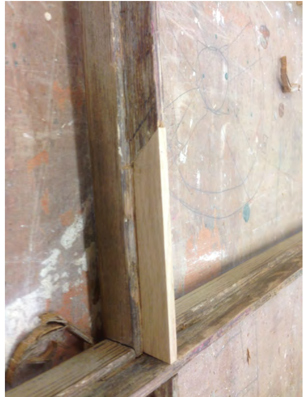
Above: Timber splice window repair. This approach ensures the historic fabric, authenticity and the essential character and appearance of a historic building/asset is retained and conserved.
