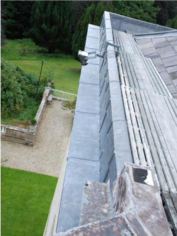
Above: Lead flashing applied to cornice and parapet upstand to protect stonework from weathering and effects of water ingress.
