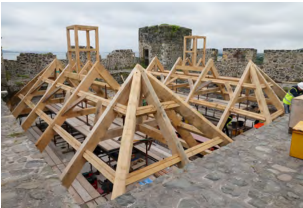
Above: Construction of a new Irish oak hipped roof structure over the Great Hall, Carrickfergus Castle, replacing an earlier 1930's flat roof. The roof design, informed by extensive research and onsite investigative works has sensitively conserved the asset and enhanced the quality of space within the Great Hall. Image 1: During Construction. Image 2: View of new exposed roof structure from inside the Great Hall.
