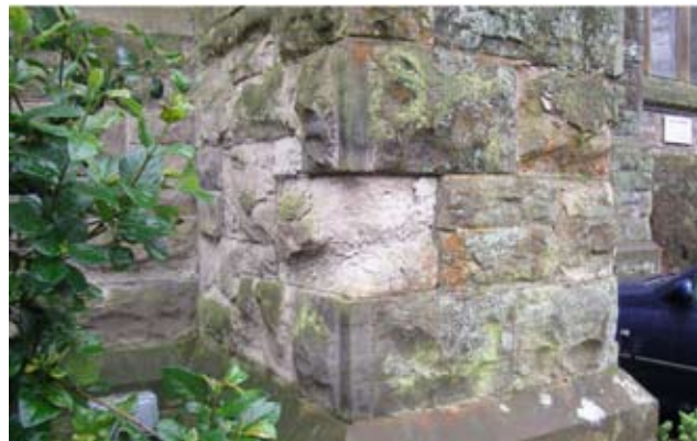
Proximity of shrubs to a building, particularly on north facing aspects where more humid conditions naturally occur, can slow drying of masonry and exacerbate deterioration.
