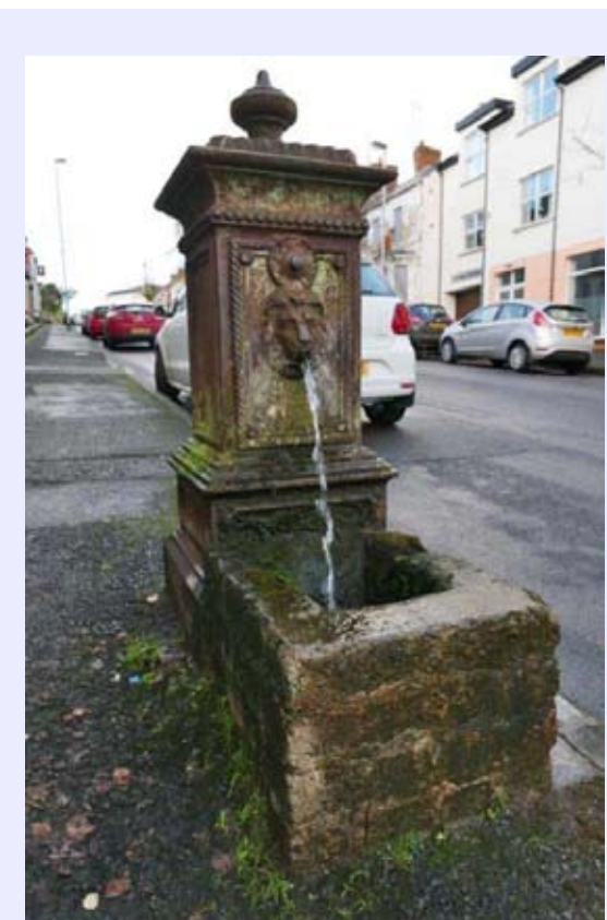
A rare surviving cast iron water fountain dating from c.1870 by engineering firm Glenfield Company Limited was listed in Waterside, Coleraine. Square on plan with ornate decoration including a distinctive lion-head surround to the spout, typical of that used at this time. Of interest as it predates mains water installation and is thought to have drawn spring water – according to locals the water had healing qualities. Significant from a social perspective, drinking fountains were prevalent in the late Victorian era as the only supply of fresh water for many people.
