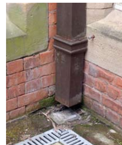
Something as simple as litter blocking a drain cover can slow the removal of excess water during heavy rainfall events and, if left unattended, can contribute to increased moisture loading of masonry materials.
