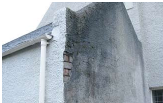
The Hill House in Helensburgh, Scotland, designed by Charles Rennie Mackintosh and built in 1902. Cracking of inflexible cement render caused by expansion of underlying masonry materials. This enables moisture to enter the structure where it is held because of the lack of breathability in the cement render, thereby leading to problems of damp in the building’s interior.
