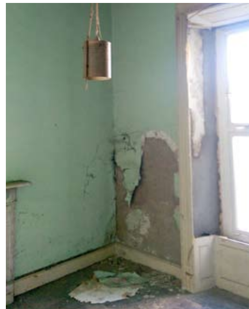
The rising damp and timber decay industry frighten homeowners with red flashing moisture meters and often recommend destructive damp proofing treatments.
