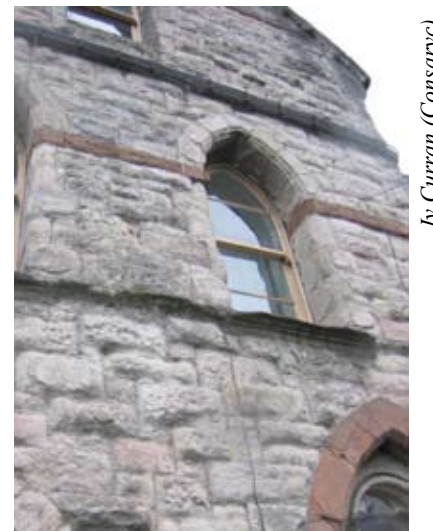
Severe weathering-related loss of definition of cills and stringcourses over time lessens the loss of excess moisture being shed via drip-fall and allows it to remain on masonry surfaces where it can be absorbed and increase the moisture load of the stone.
