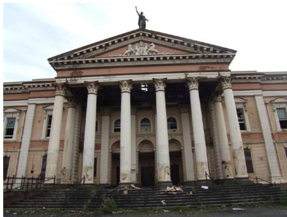
Crumlin Road Court House falling into further decay while currently held in development limbo.
