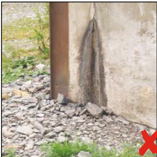
Photo 6 - Leaking silage clamp
