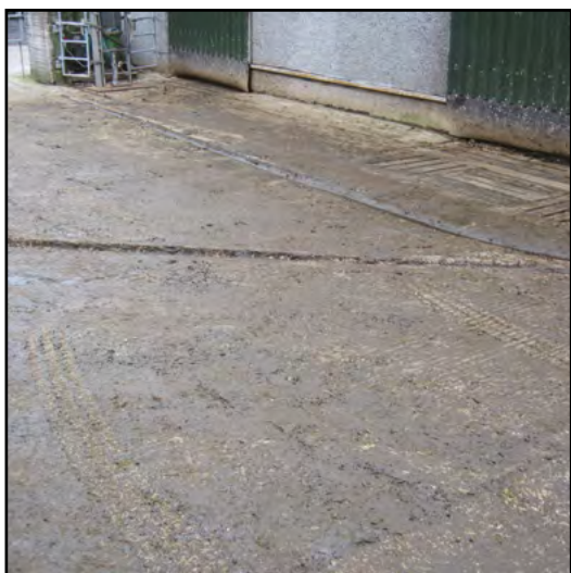
Photo 27 - Run-off from a frequently used collecting yard is slurry.
