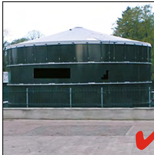
Photo 11 - Well maintained above ground slurry tank
