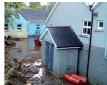
Plumbridge: the Parish Hall showing tidemark and damage after extensive flooding due to severe weather – August 2017.
