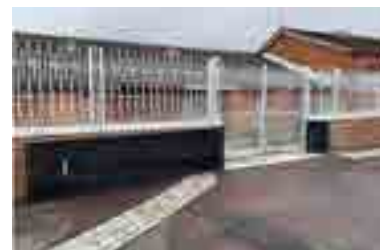
Brick-clad reinforced concrete flood wall with bespoke railing to match original + Flood gate
