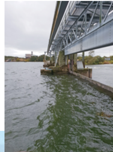
Below & Right: The Sluice Gates at Toome are used to control water levels within Lough Neagh
