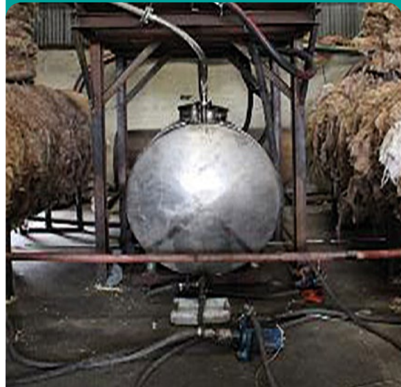
Photo of a fuel laundering plant
