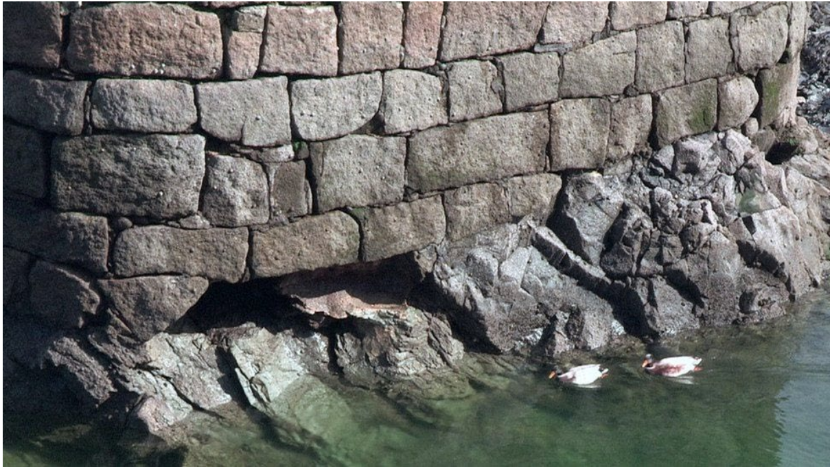
FIGURE 12. DAMAGE TO ANNALONG HARBOUR WALL
