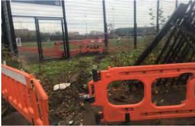
Criminal Damage at the Centre caused via dangerous driving in November 2017
