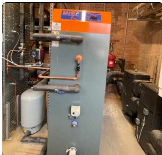
Solar Assisted Heat Pump installation in an older building on the Knockbracken Healthcare Park.
