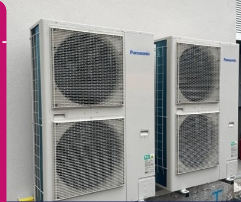
Double Stacked Air Source Heat Pumps
