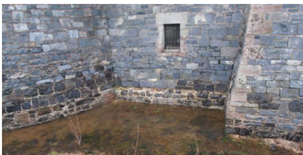
Extreme case of water not draining from building perimeter; in this case due to a broken culvert, water is able to soak into the wall
