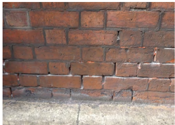
Mortar washout at the base of a wall
