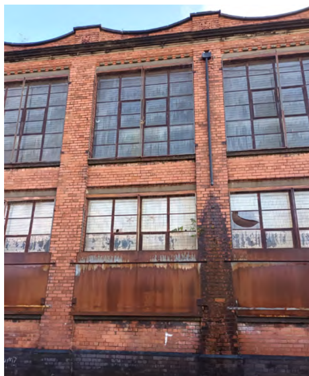
Missing downpipe which has caused damage and staining to the brickwork, and wall saturation
