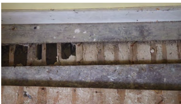
Floor with parging to underside of boards, discovered on opening up
