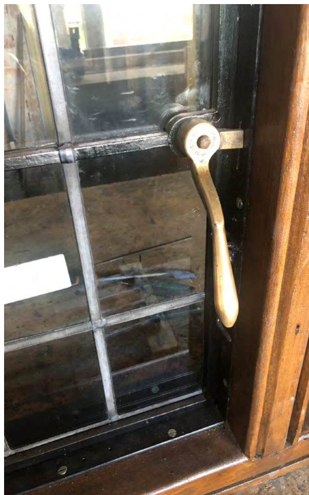
Protruding historic stay
