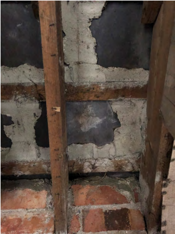
Parging/torching to underside of slate
