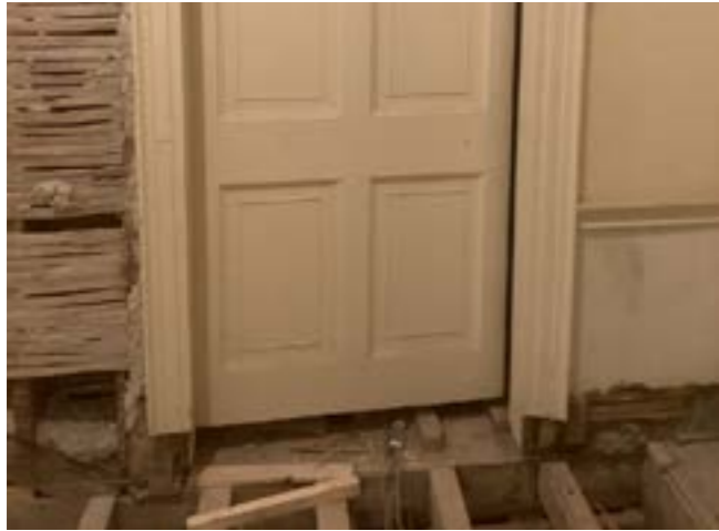
Door with surrounding floorboards and plaster removed showing gaps in walls, floors and door frames that need passive fire protection design to adequately firestop them
