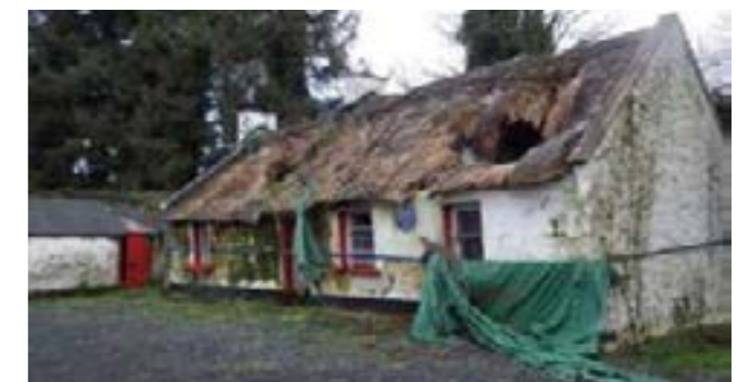
The listed family home of the renowned Irish 19th century novelist and writer William Carleton, complete with 'blue plaque'. William Carleton's Cottage, Clougher (HB13/02/004) (Image Source: HED 2022 - one of many such examples of thatch at risk within that eye-opening report)
