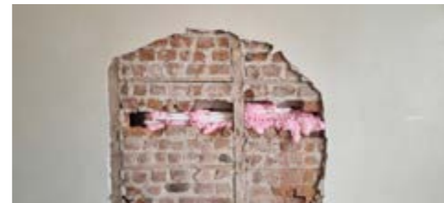
Plaster removed exposes a hole incorrectly firestopped, typically carried out by an inexperienced installer
