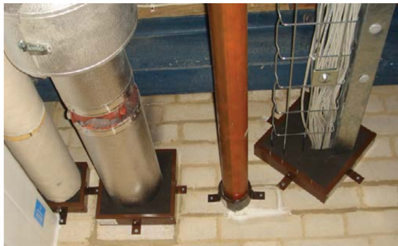
Services with intumescent collars installed at compartment wall
